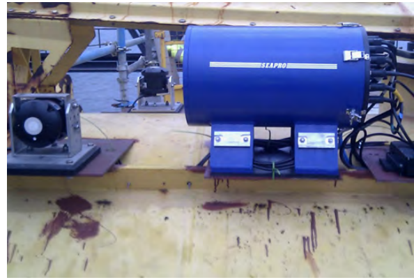
(b) Instrumentation and instrumentation control-box installed on the 500KW machine
